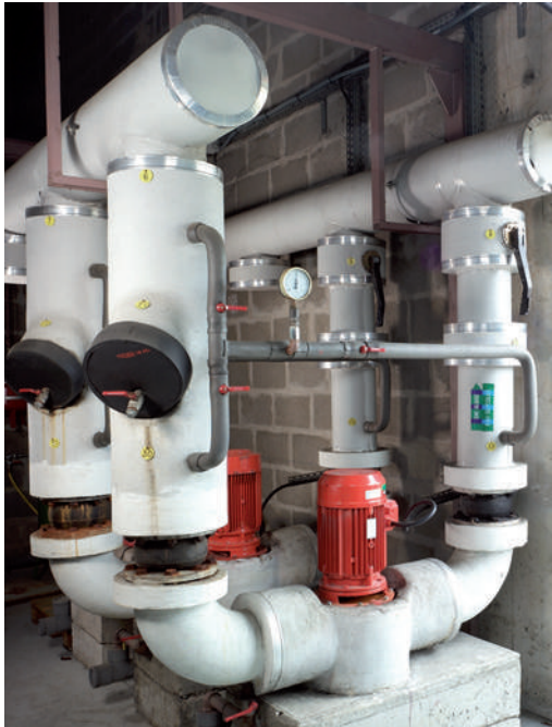
Example of using the Altistart 22 soft start/soft stop unit in a pumping application
