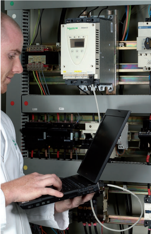
Testing and start-up of the ATS 22 soft start/soft stop unit using SoMove setup software
